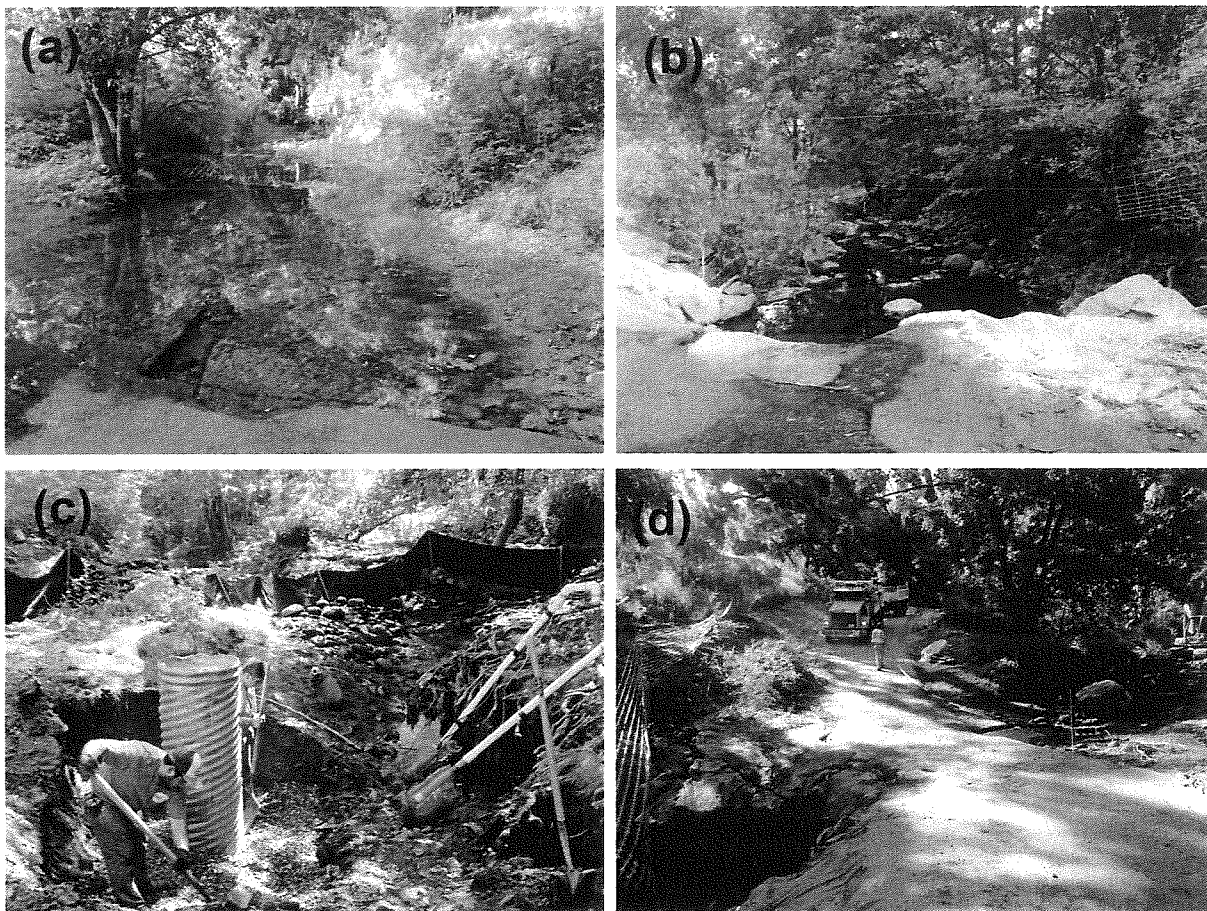
Figure 1: Dewatering of the Quiota Creek Crossing 2 project site on 9/6/11 looking (a) upstream and (b) downstream before dewatering, and (c) upstream and (d) across the crossing after dewatering.
