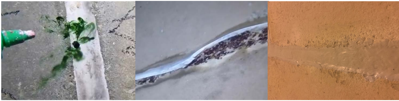
Figure 3. (left) Food grade dye utilized to locate leaks; (middle) joint caulking and oakum separating from the joint; (right) repaired and re-caulked joint.
