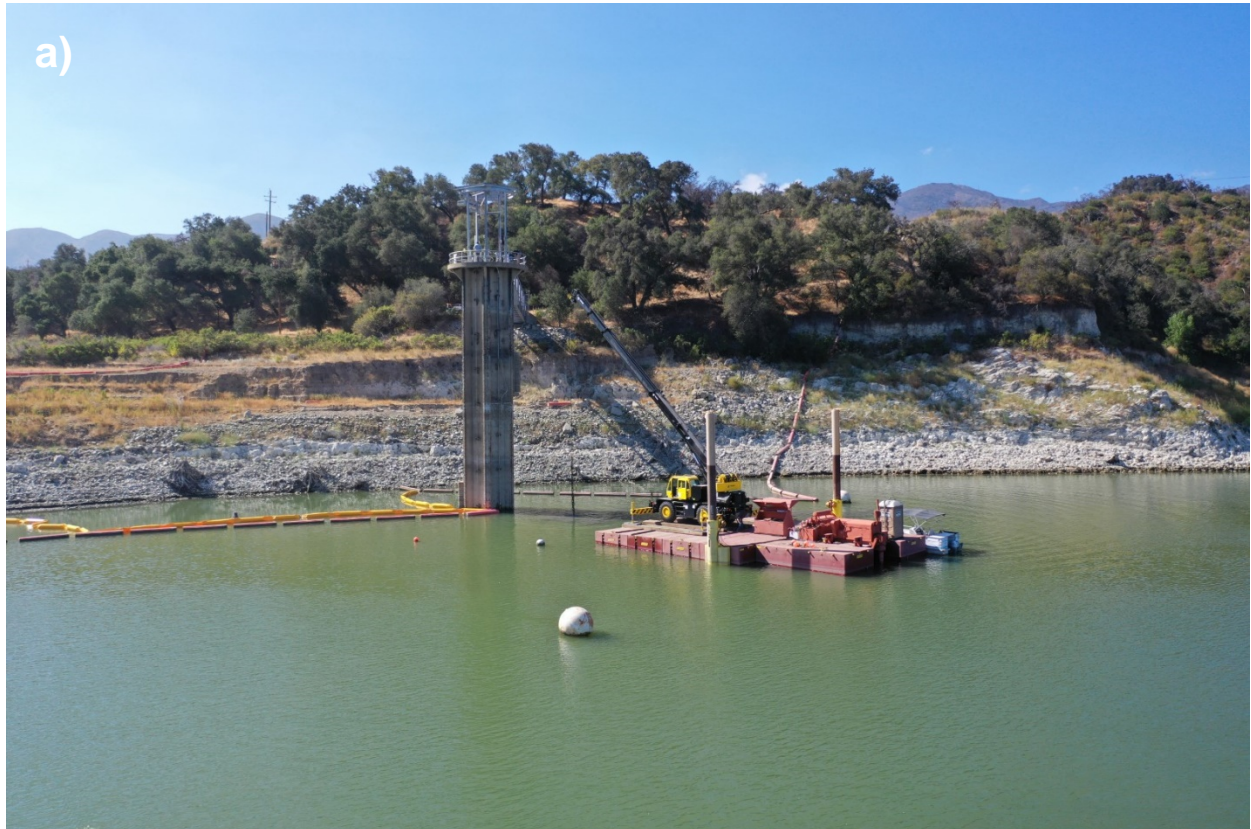
Figure 2: a) work barge dredging around the intake tower; b) clamshell bucket utilized for dredging around the berm and around the intake tower; c) airlift utilized for finer scale dredging around the intake box.
