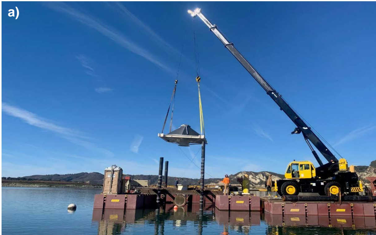
Figure 8: a) intake screen being lifted and installed on intake screen piles; b) intake screen with 90 degree elbow being assembled above water pipeline and then lowered down to bottom;
