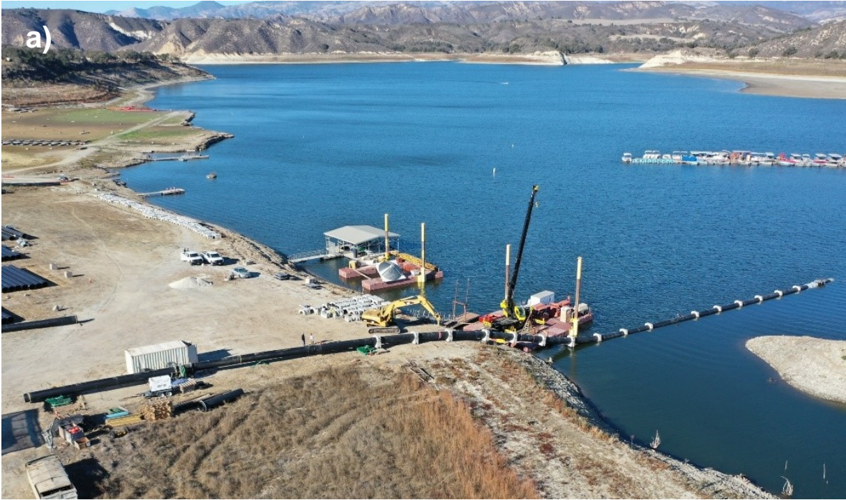
Figure 4: a) HDPE pipeline being fused, concrete weights installed, and being pushed out into the water; b) concrete anchor weights installed on pipeline
