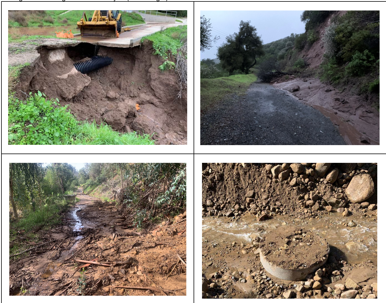
Figure 2. Overview of damages caused by the January 9-10 storms including the Lauro Reservoir access road washout (top left), Glenn Anne access road landslide (top right), Sycamore Canyon minor slides (bottom left), and blowoff structure damage and missing lid at Toro Canyon (bottom right)
