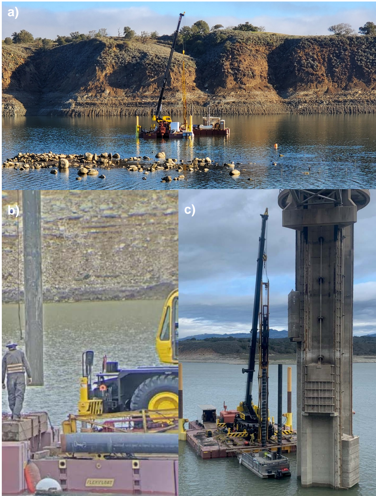
Figure 7: a) pile driving the four 12-inch steel piles for the intake screen; b) setting the 16-in holdfast piles near the intake screen into the pile driving template; c) driving the two 16-in hold fast piles near the North Portal Intake Tower
