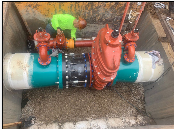
La Mirada Piping and Valve
