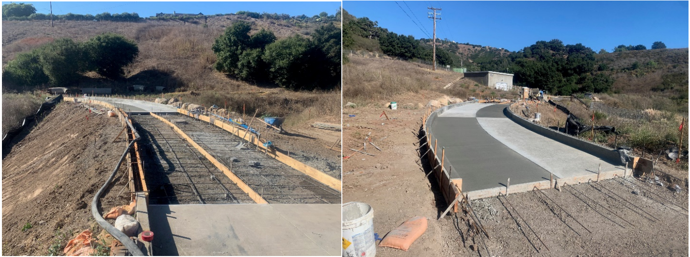
Figure 2. Lauro Reservoir Bypass Channel Road Repair - (a) washout and cantilevered concrete channel and manhole after 2023 storm event; (b) backfill and compaction of washout; (c) forms and rebar for replacement concrete channel; (d) concrete channel extension poured to mitigate for future damages.
