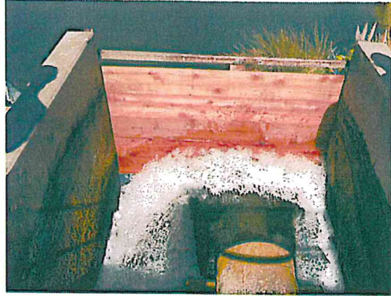
Stop Logs (After)
