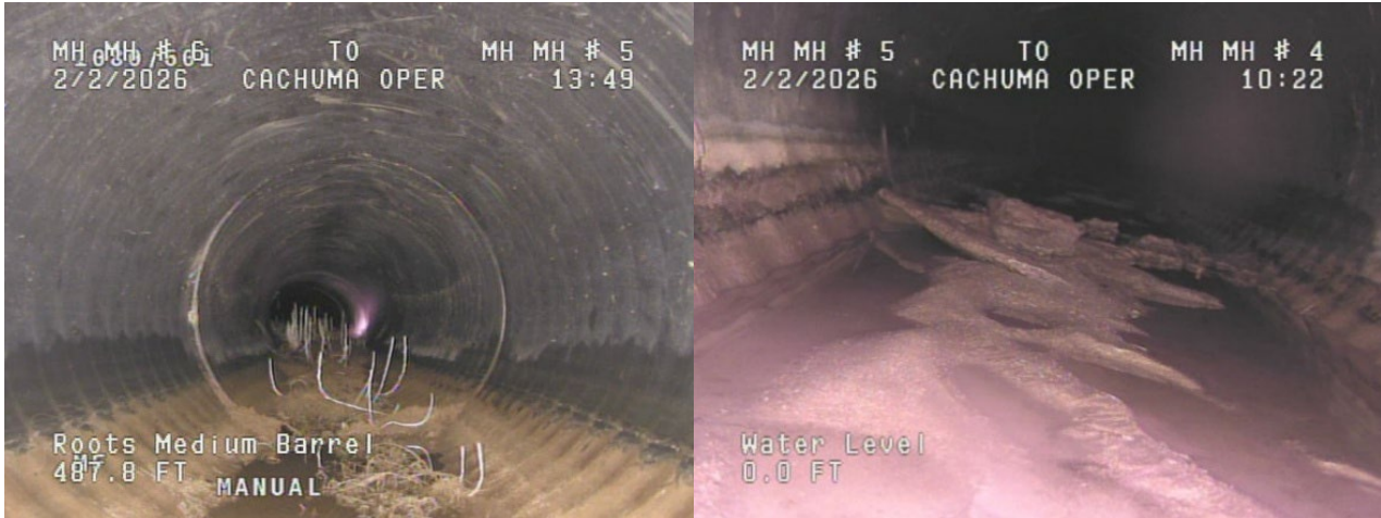
Figure 1. 24” Lauro Reservoir Storm Drain – root intrusion on left, sediment on right
