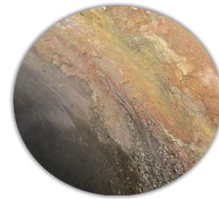
Figure - Concrete Lining Deterioration within the Tecolote Tunnel
