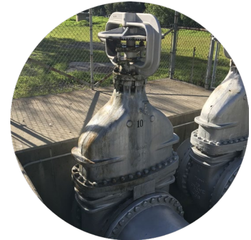
Figure – Lauro Control Station Gate Valve
