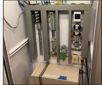
SCADA Control Panel
