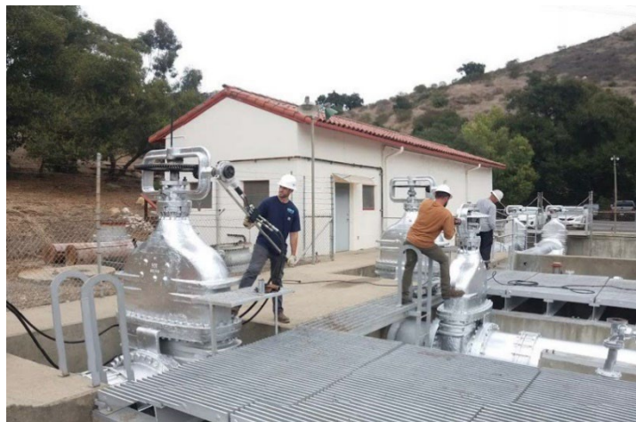
Lauro Control Station Valve Exercise
