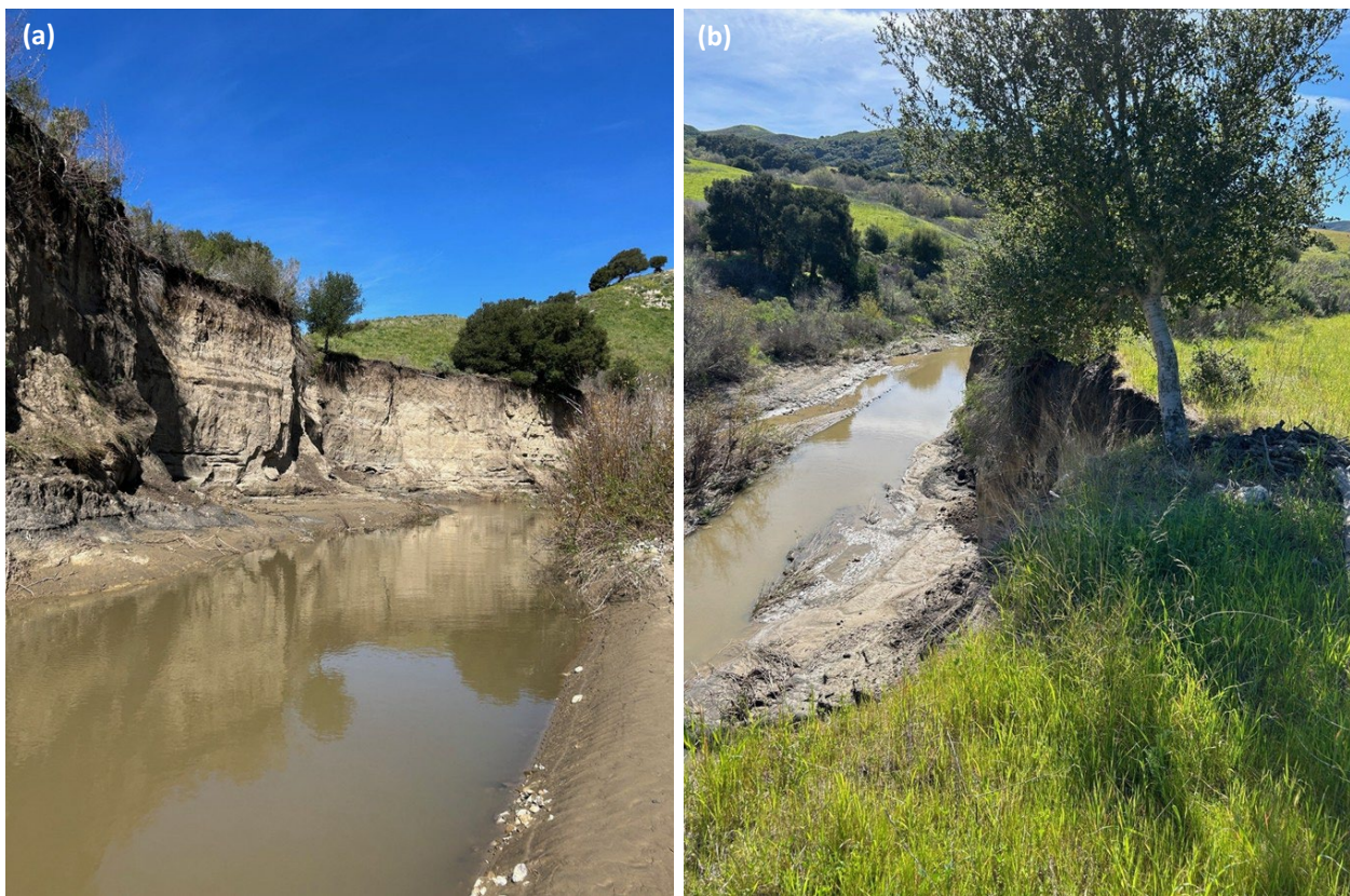
Figure 2: Downstream bank condition in February 2026 looking (a) upstream and (b) downstream.
