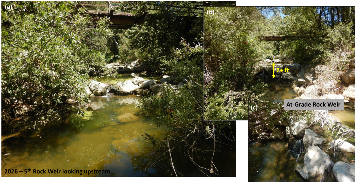
Figure 1: 2026 condition looking (a) upstream at the 5 th rock weir and the 2+ foot jump height, (b) upstream at the exposed at-grade rock weir, and (c) at the at-grade weir from the top.
