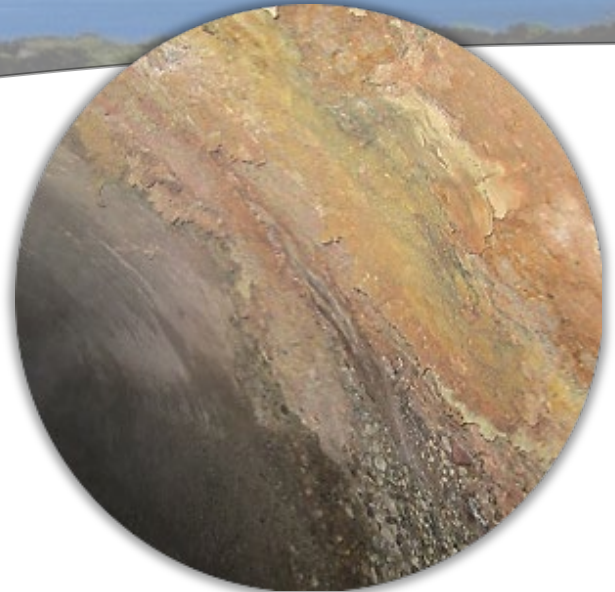
Figure A.13 Concrete Lining Deterioration within the Tecolote Tunnel
