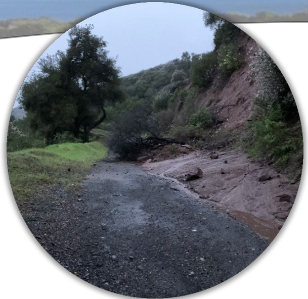
Figure A.5 Glen Annie Road Damage following January 2023 Winter Storms
