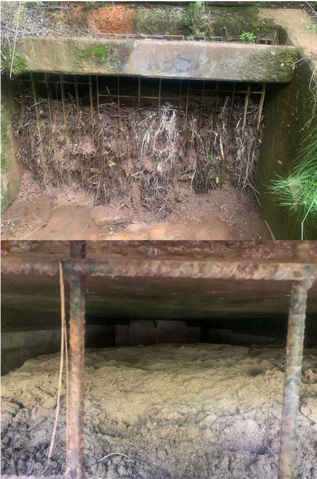
Figure 2. Sediment and woody debris in Lauro Reservoir Spillway Stilling Well
