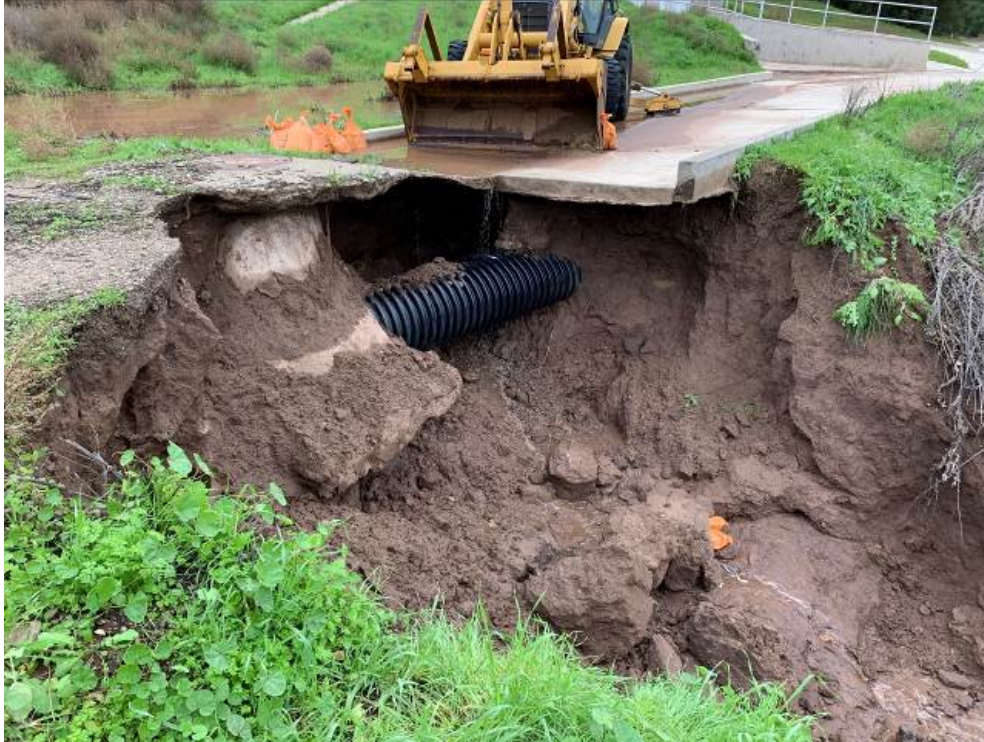
Figure 1. Lauro Reservoir Road/Bypass Washout following the January 9 th , 2023 storm event
