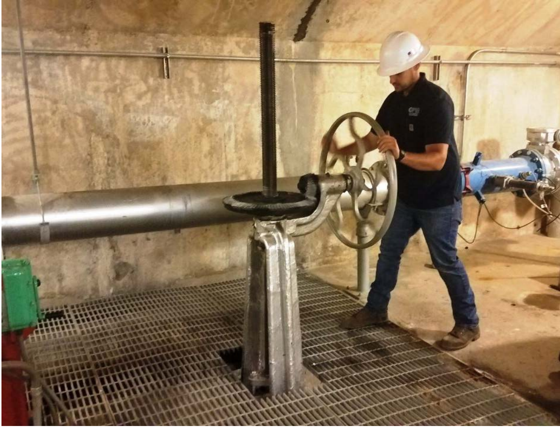
Exercising the 30" Guard Valve in the North Portal Gate Chamber
