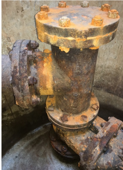
Original valve and piping in blowoff structure
