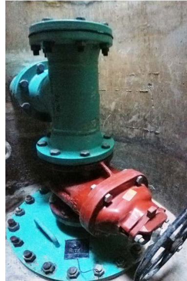
Replaced outlet, valve and piping in blowoff structure during Schedule B in 2019
