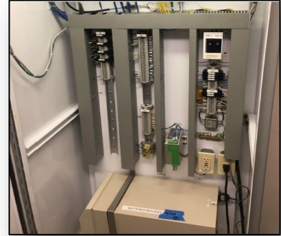
SCADA Control Panel
