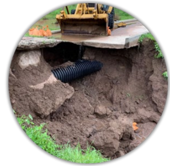
Figure - Lauro Reservoir Bypass Channel Washout January 2023 Winter Storms
