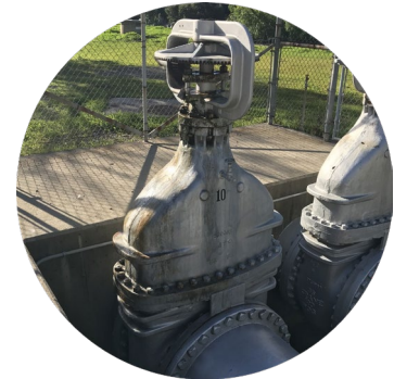
Figure – Lauro Control Station Gate Valve
