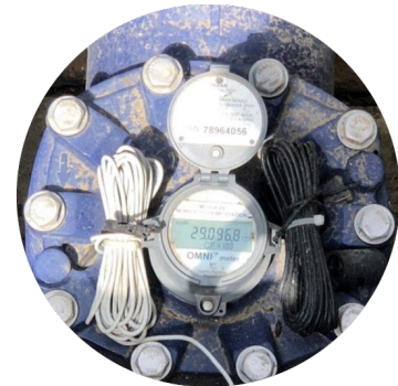
Figure – Montecito Pump Station Meter
