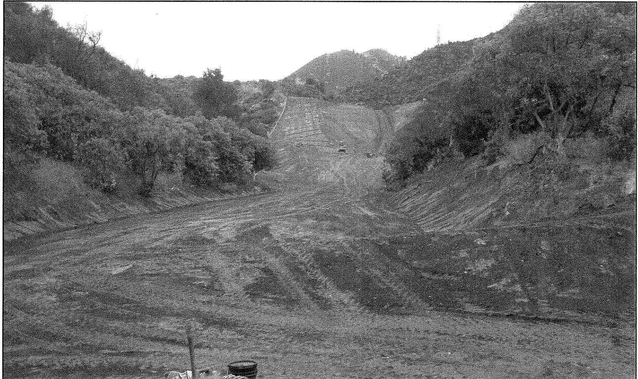
Pipeline Right-of Way has been Finish Graded and Permanent Erosion Control Placed
