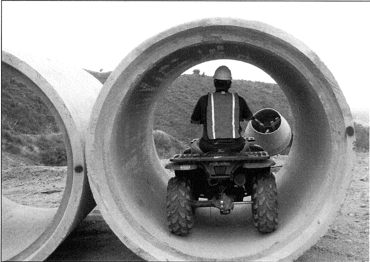
Pipe to be Installed at Junction Structure to Allow Access to Tunnel with ATV
