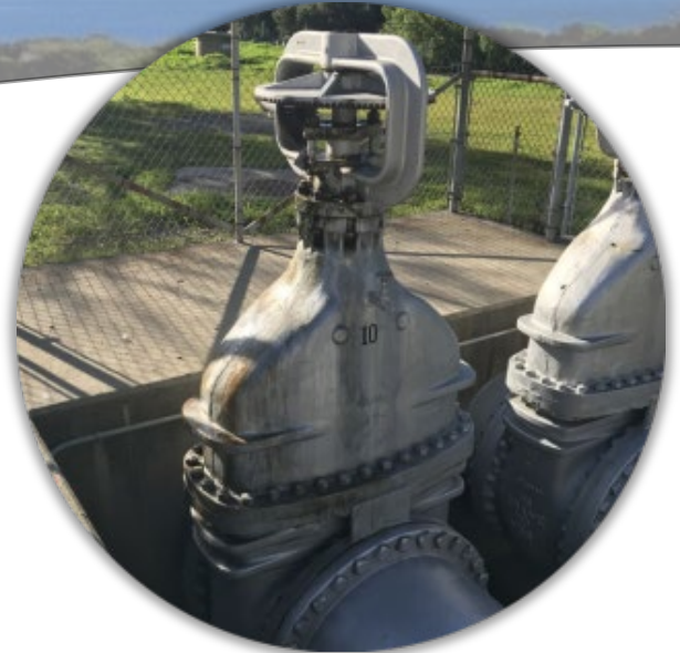
Figure A.9 Lauro Control Station Gate Valve
