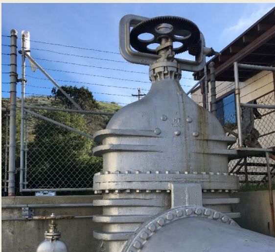
Figure 4. Lauro Control Station Gate Valve
