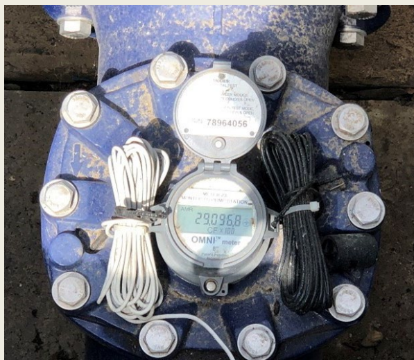
Figure 6. Montecito Pump Station Meter
