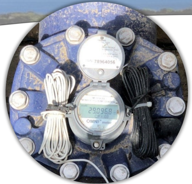
Figure A.8 Montecito Pump Station Meter
