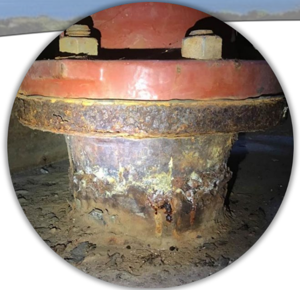
Figure A.7 Corroded Blowoff Riser Nozzle at SCC Upper Reach Station 639+50 Before Repairs
