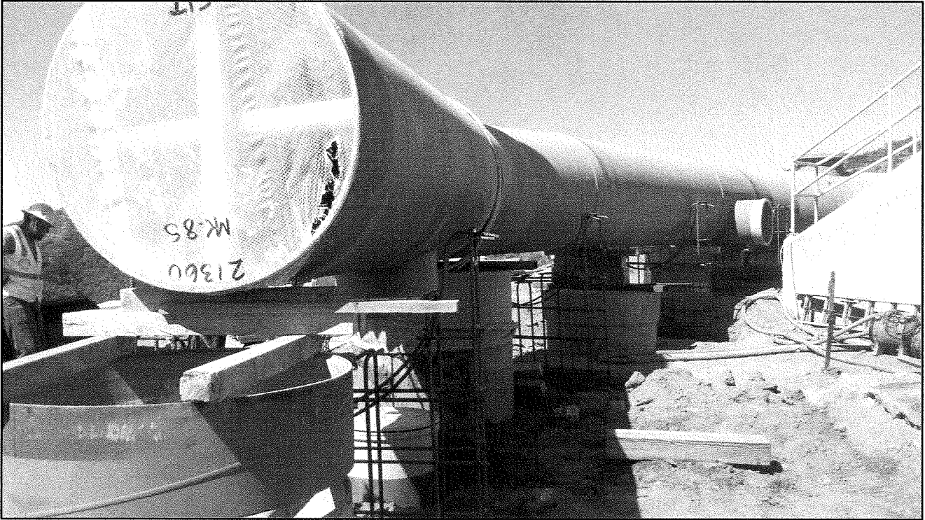
Above ground pipe at Glen Annie Turnout
