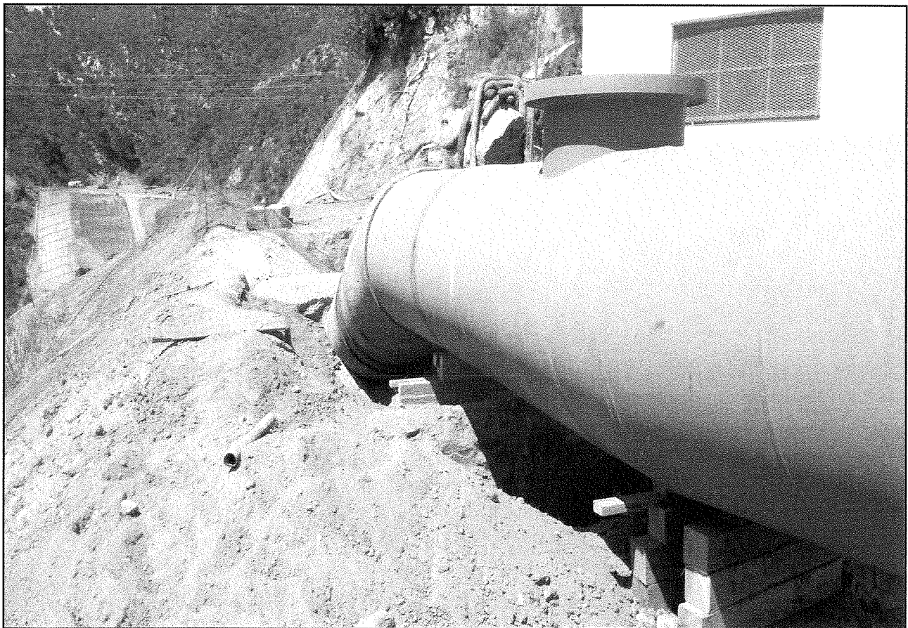
Above ground pipe at Glen Annie Turnout
