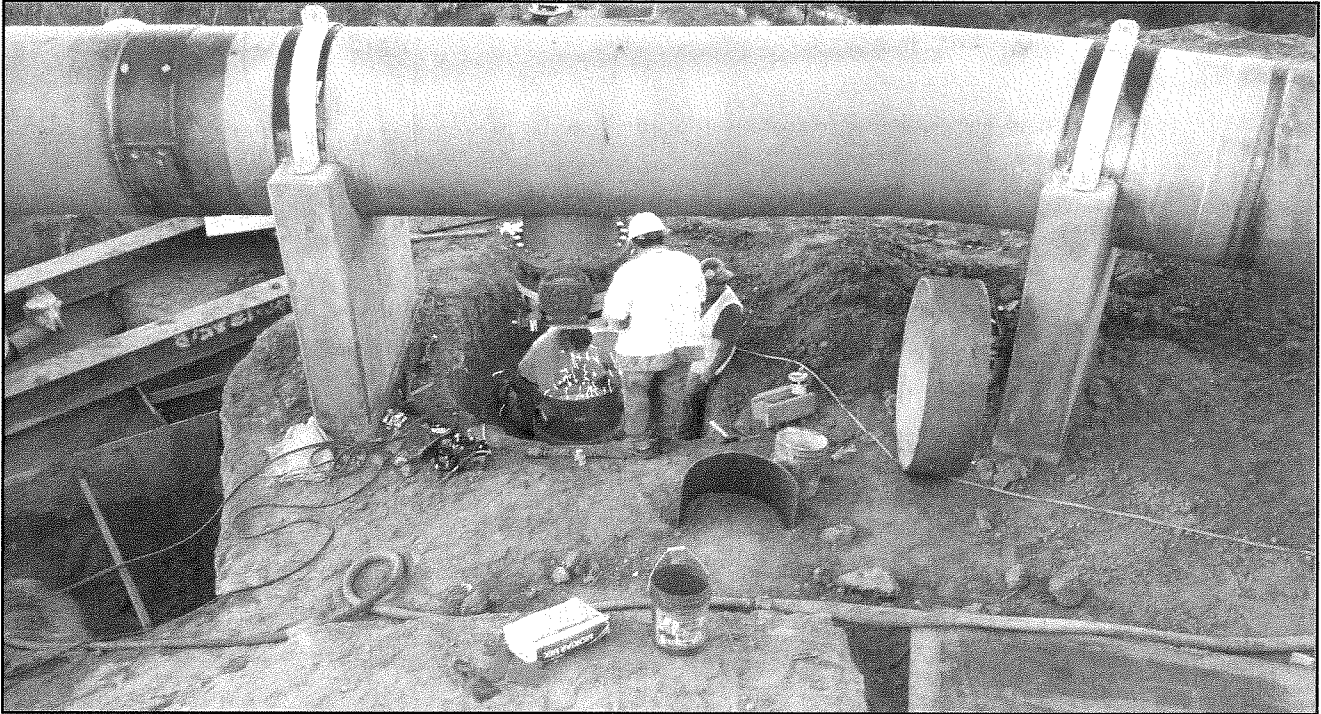
Welding up connection between new 48" pipe and existing Goleta West Pipe. Work being performed during shutdown.
