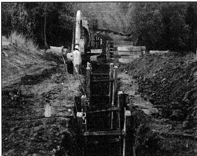
Shoring installed to allow men in the trench to compact sand bedding
