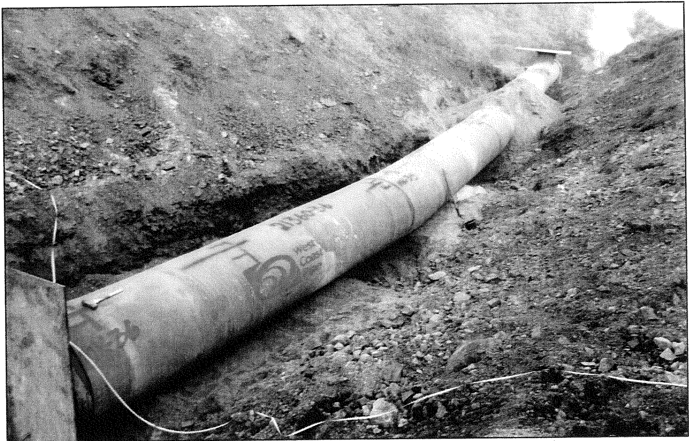
Pipe cresting the slope at the plateau. Note Tee for air release valve
