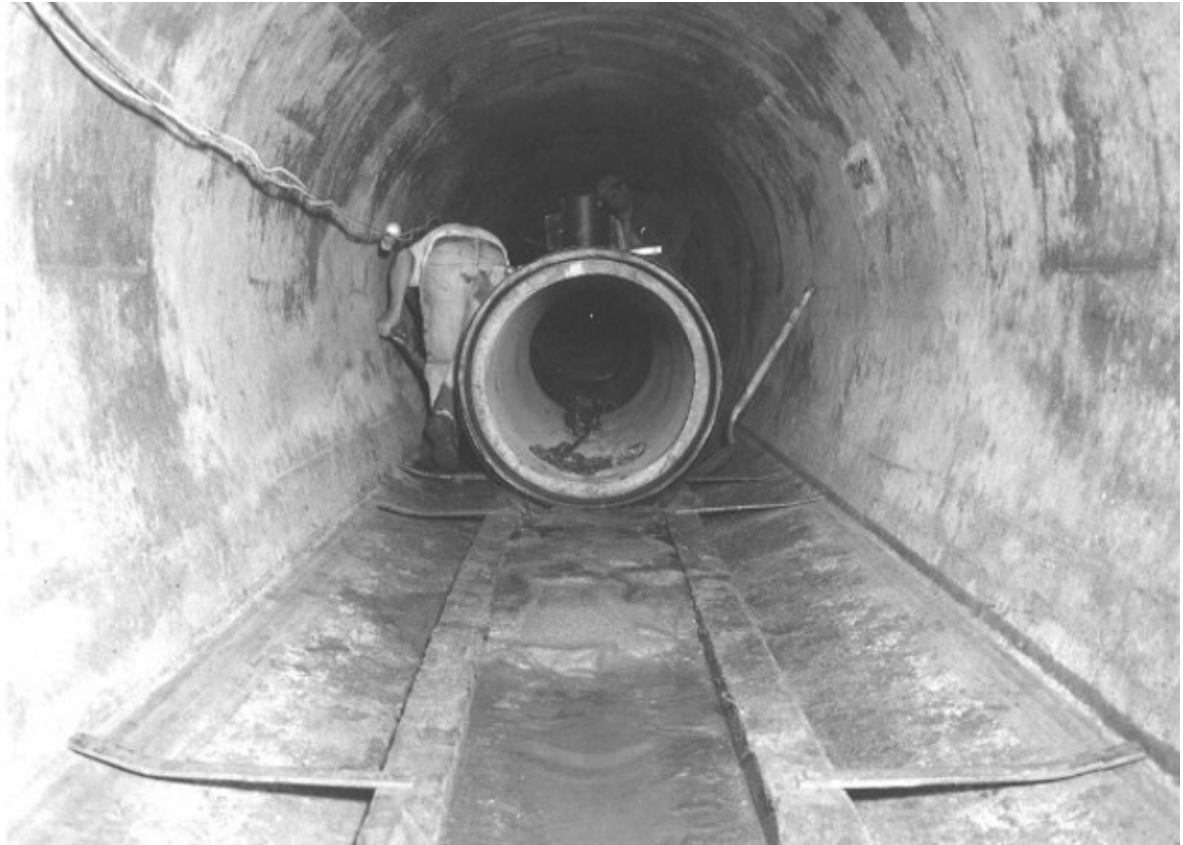
Figure 1. Historical photo from April 25, 1953, showing the 30-inch I.D. South Coast Conduit within the horseshoe-shaped Sheffield Tunnel
