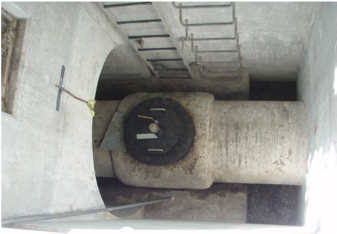
Figure 3. Layout of the Sheffield Tunnel East Portal as viewed from above. The Project would include a bypass line connection flange into the vault above the existing SCC.
