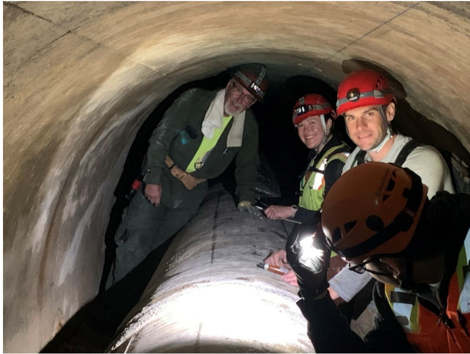
Figure 2. Photo of inspection in April 2025, showing the cramped working space in the 6-ft diameter tunnel with a 3-foot outer diameter concrete pipeline.
