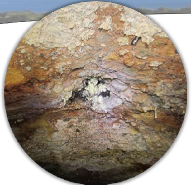
Figure A.12 Clogged Weep hole in Tecolote Tunnel
