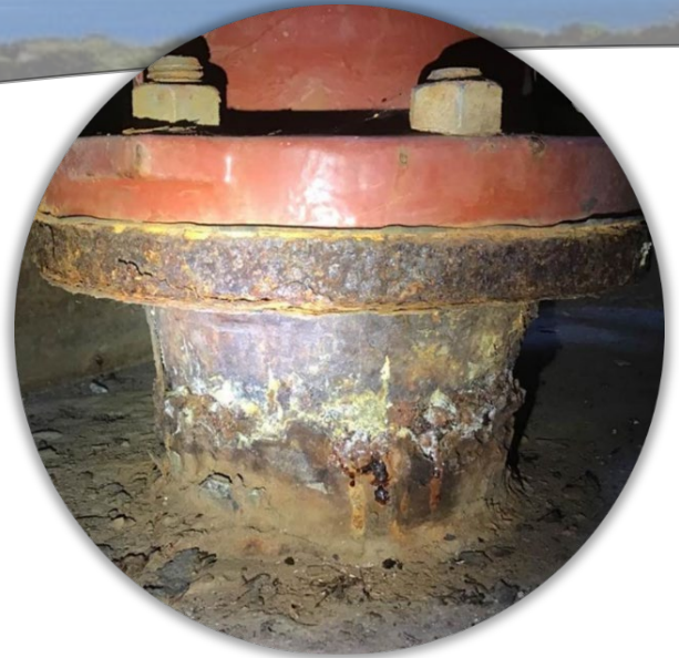
Figure A.7 Corroded Blowoff Riser Nozzle at SCC Upper Reach Station 639+50 Before Repairs
