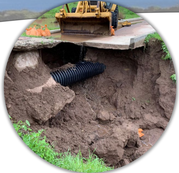
Figure A.4 Lauro Reservoir Bypass Channel Washout January 2023 Winter Storms
