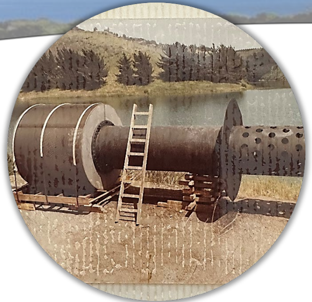
Figure A.6 Intake Structure Extension to be Placed in Lauro Reservoir April 5, 1981
