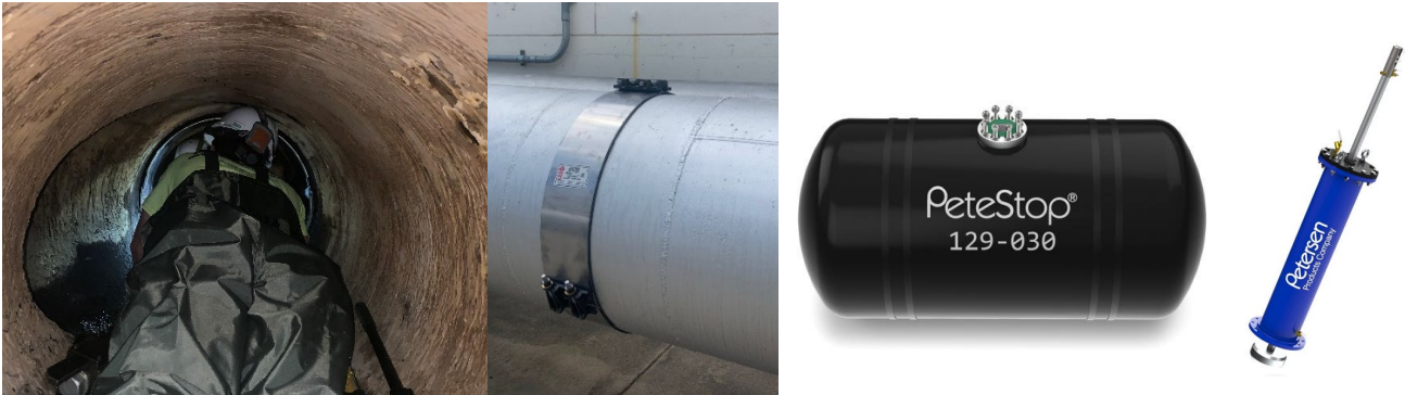
Figure 1: Planned Emergency Repair Options (left) internal Hydratite seal being installed in Ortega Reservoir Outlet Pipe in 2022 – which is same size and type as Sheffield Tunnel pipeline; (middle) three part external repair clamp with removable lugs tested on 36” OD pipeline; (right) inflatable plug stop with insertion device that would be bolted on to SCC air vent structure to allow temporary activation of the Stanwood intertie.
