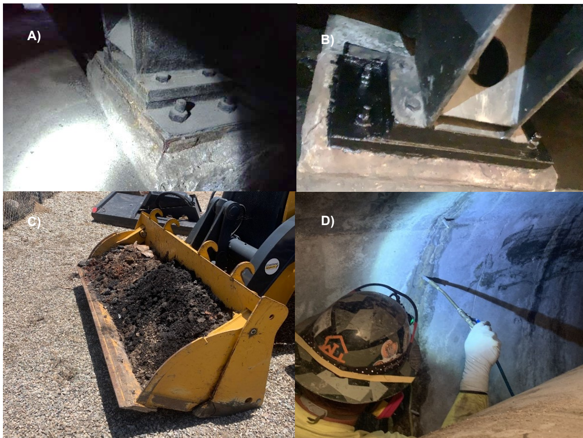
Figure 2. Lauro Outlet Works Tunnel Work – a) corrosion on pipeline support base plates pre-work; (b) cleaned and re-coated baseplates; (c) mineral deposits and iron- and manganese oxidizing bacteria deposits removed from tunnel invert; (d) injection of leaks in tunnel was with water stop grout.
