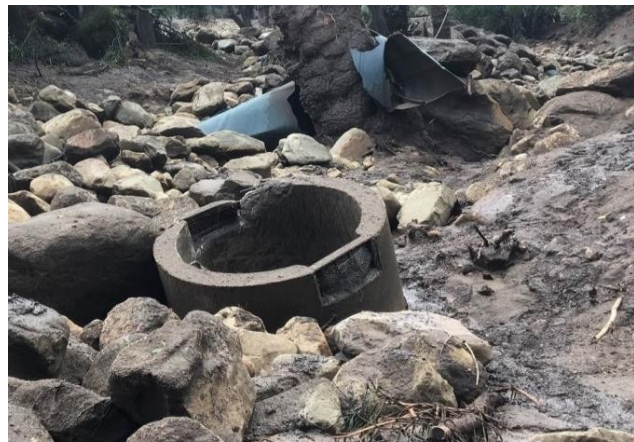
Damage to SCC vault after 1/9/18 debris flows
