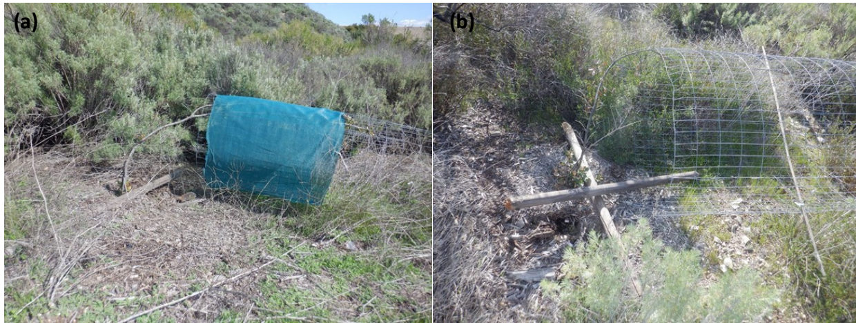
Exhibit 1: Long Pool Secondary Flat wind damage showing (a) & (b) toppled infrastructure and trees.
