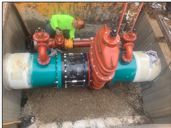
La Mirada Piping and Valve
