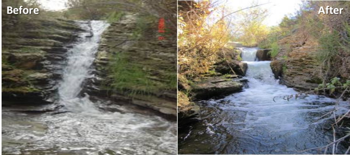
Figure 72: Fish passage and habitat restoration at Hilton Creek at the Cascade Chute Project that was completed in 2005.
