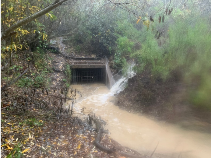
Lauro Spillway Stilling Well flowing freely during peak of Dec. 21 storm. Side cascade was investigated and originated from a culvert upslope
