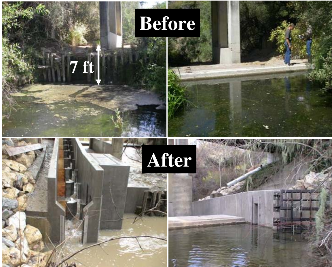
Figure 50: Fish passage and habitat restoration in the fall of 2008 at Rancho San Julian on El Jaro Creek.
