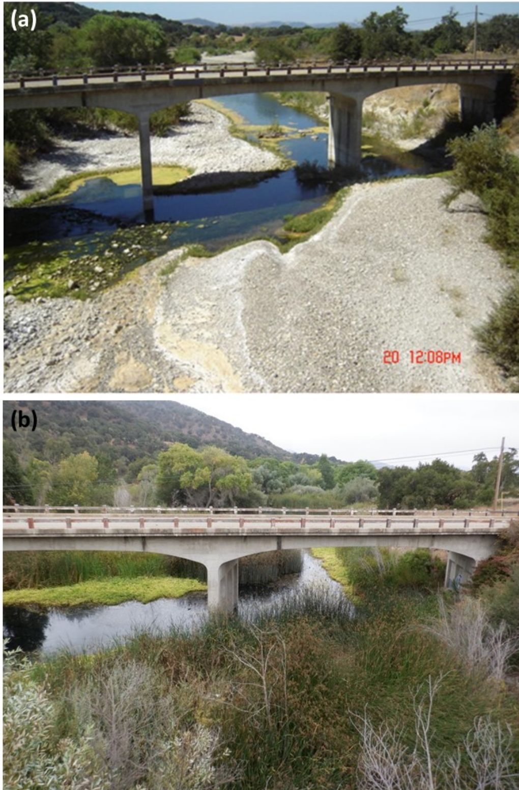
Figure 58: Photo points (M-6) collected at Highway 154 Bridge looking downstream in (a) September 2005 and (b) September 2021.
