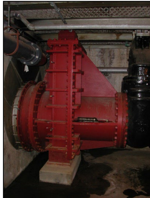
North Portal Jet Flow Control Valve
