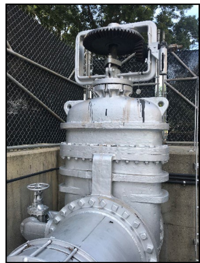
Sheffield Control Station Valve
