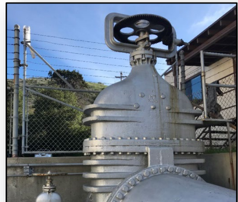
Lauro Control Station Valve
