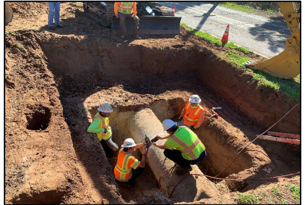
La Mira Isolation Line Valve (Installed 2022)
